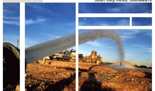
Hydraulic testing fire ring South Corp Wines, Coonawarra
